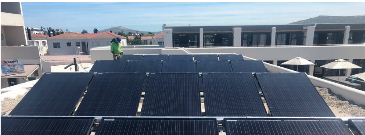
High-temperature PVT system at Windtown Hotel in Langebaan, South Africa. 27.5 kW thermal and 7.6 kW electrical combined with a 19 kW heat pump
